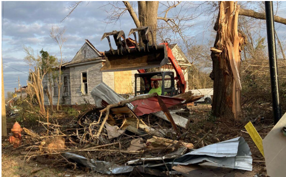
Crews work to cleanup storm debris from January 12th tornado in Selma. Source: selmasun.com/news (5/2/2023)
